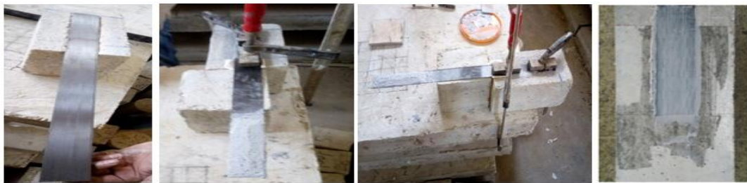
d. CFRP Surface preparation e. Adhered CFRP to concrete f. Supported CFRP
