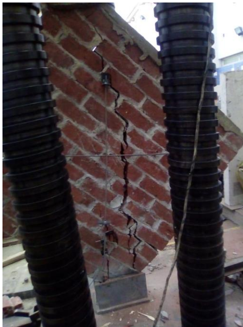
Fig1 (c):Cracking Pattern and failure mode
