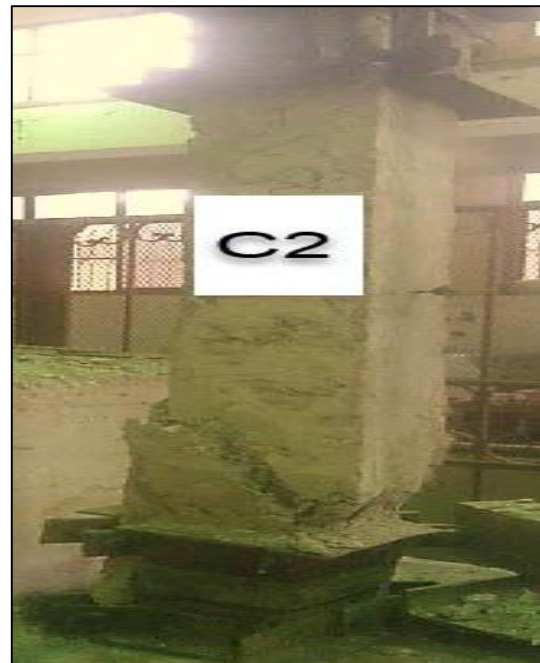
Fig. 8. Failure mode of Specimen C2
