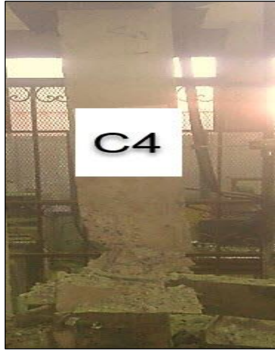
Fig. 10. Failure mode of Specimen C4
