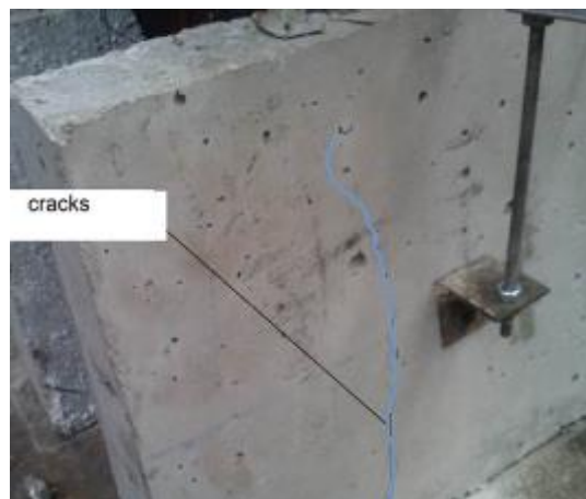
Figure (13): Failure of push-out specimen (P2)
