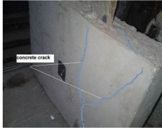
Figure (15): Typical cracking mode in push-out test specimen (P4).
