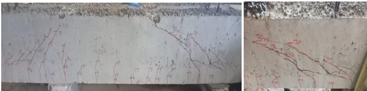
Fig.14: Crack pattern of beam SCC-B3 after shear failure
