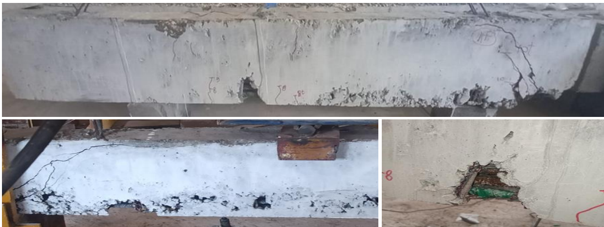
Fig.13: Crack pattern of beam NVC-B1 after failure
