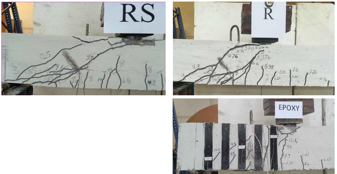
Figure 3: cracks pattern for all specimens
