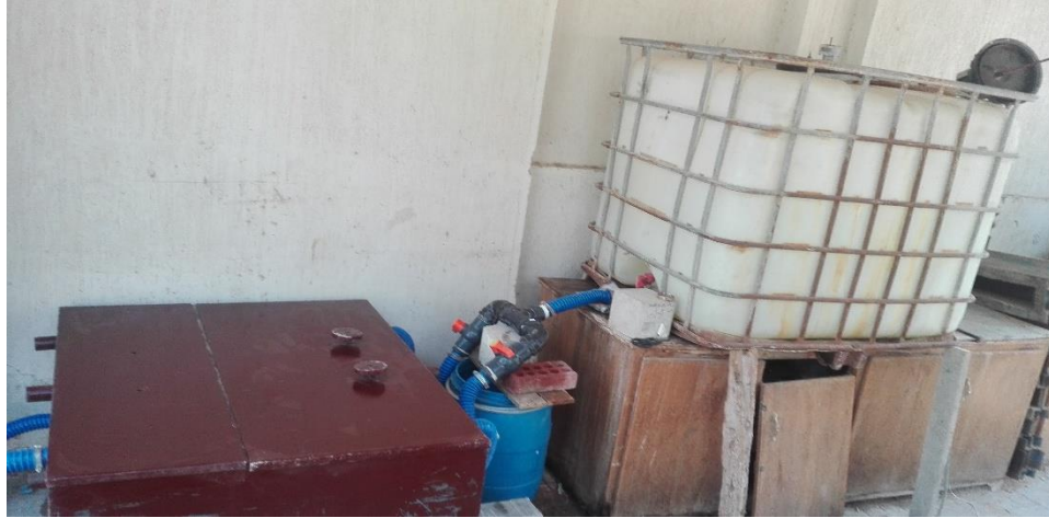
Figure (1) Pilot unit in site
