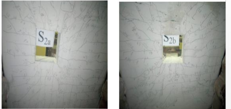
Fig. (5): The crack pattern of tested specimens s2a and s2b
