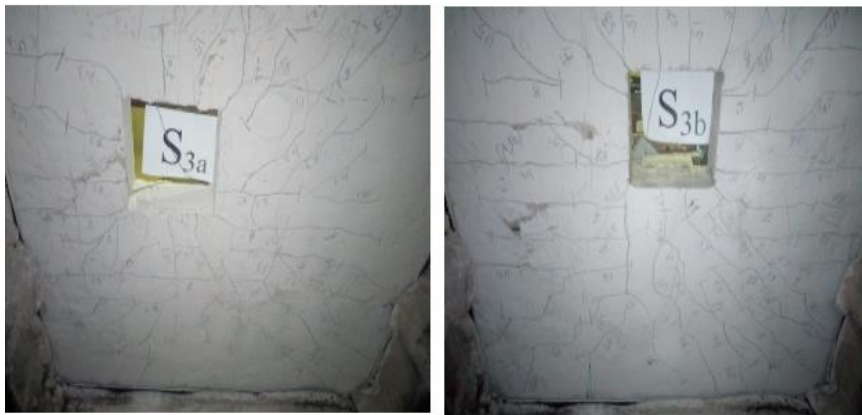
Fig (7) :The crack patterns and mode of failures ( S_{3a} , S_{3b} )
