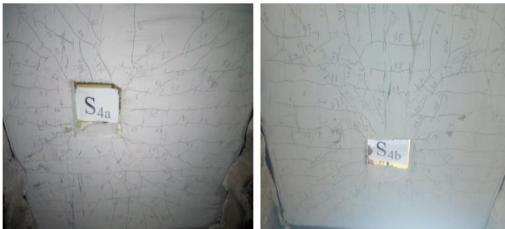
Fig (9) the crack patterns and mode of failures ( S4a, S4b )
