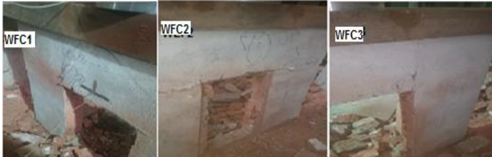
Fig. 9: Failure mode for walls strengthened with ferro-cement layer
