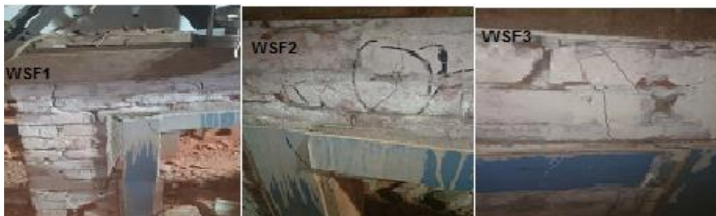
Fig. 7: Failure mode for walls strengthened with GFRP strips
