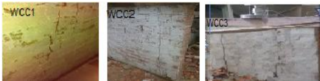
Fig 5. Failure mode of closed control wall WCC
