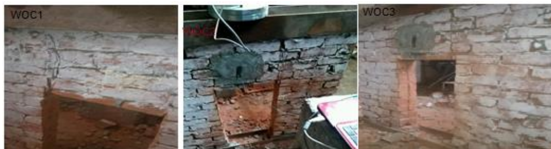
Fig 6. Failure mode of control walls with openings WOC
