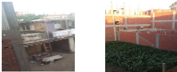
Fig. (2) Replacement Mud Brick Building with RC frame With Infill Masonry wall
