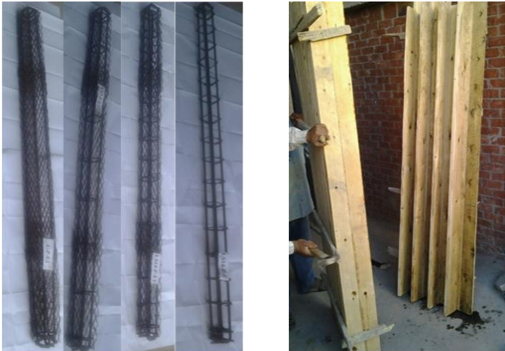
(a) Reinforcement of column specimens (b) Formworks for column specimens Fig. 2: Preparation of Column Specimens.
