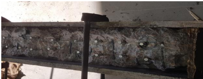
Fig.1: Studs in the old concrete before casting the new concrete cover of B5
