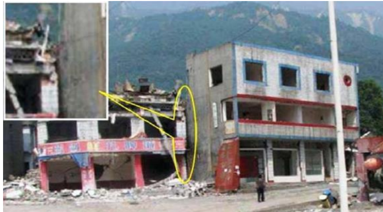
Figure 1: Pounding occurred during 12 Dec 2008, Wenchuan Earthquake, the two structures collided due to torsional vibration.
