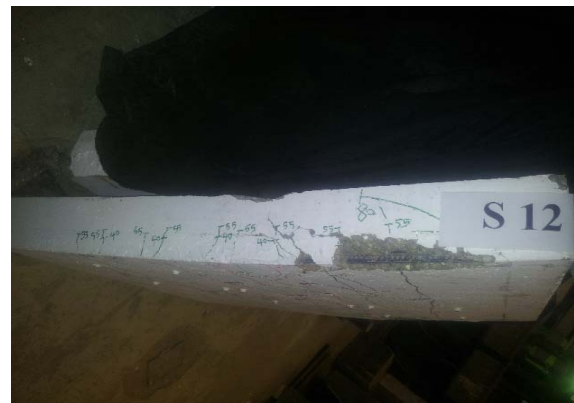
Figure 15: Shear cracks of specimen S12
